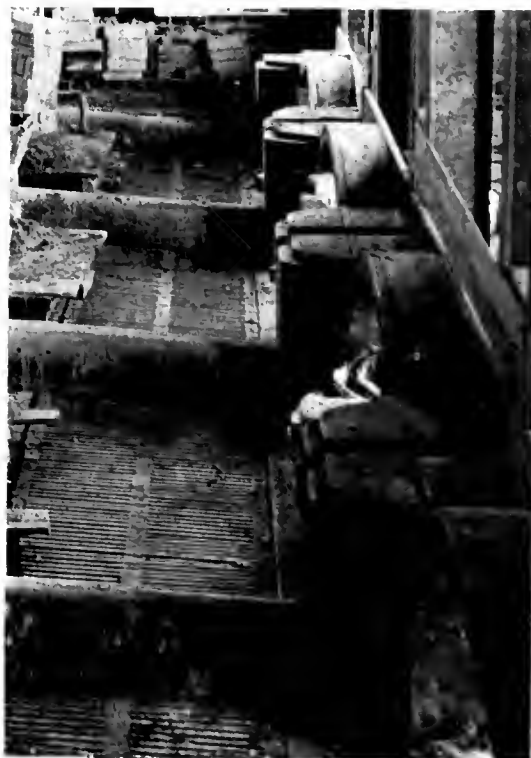
Each furnace contains four cells with low dividers between each grate, making practically a continuous grate furnace.
